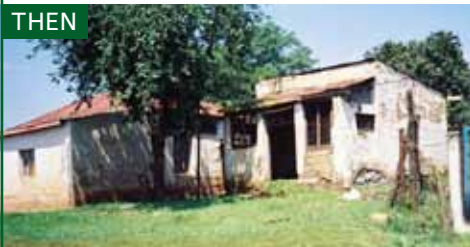
► Bonginkosi School then – a hazardous collapsing building with minimal facilities.
